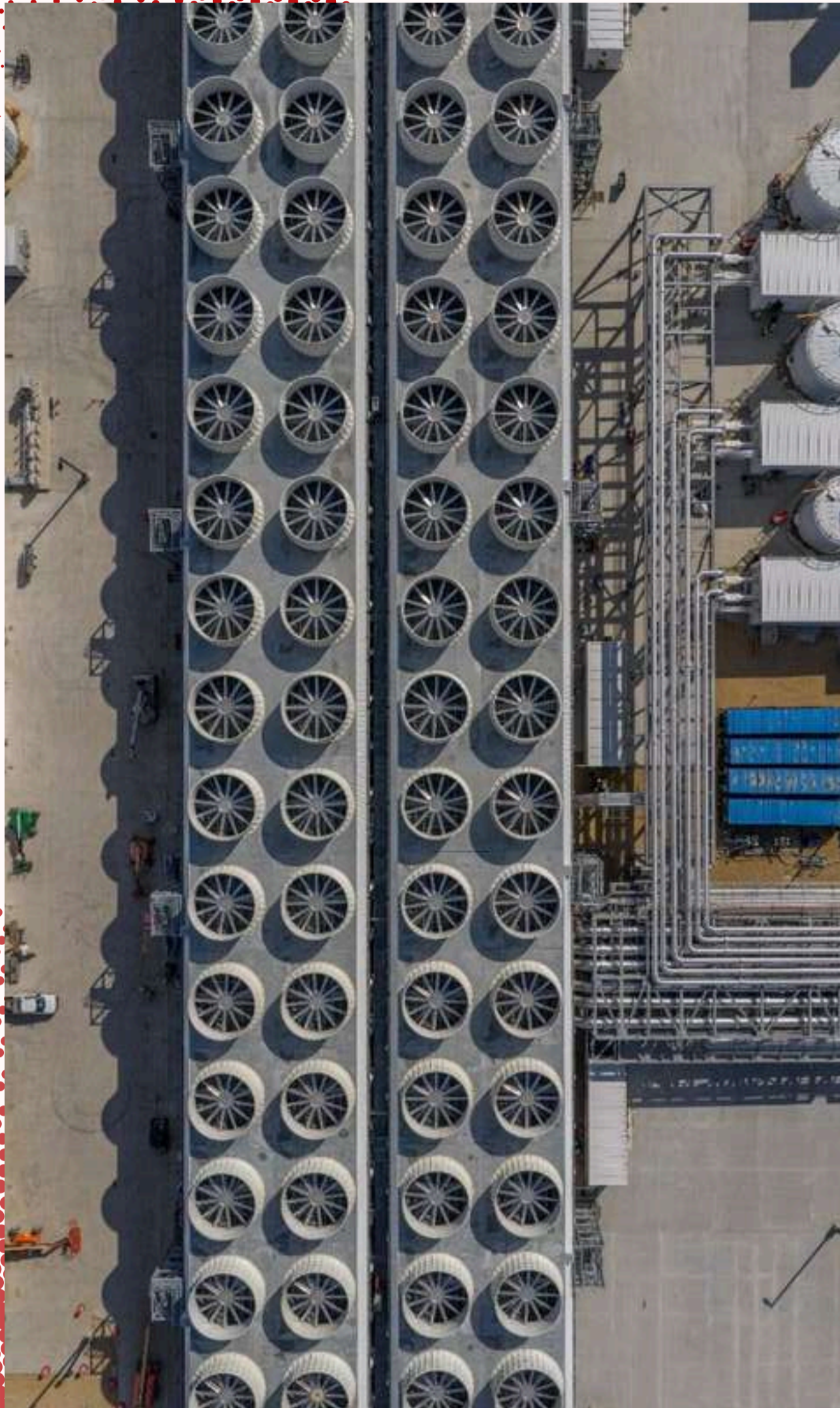
Aerial view of part of the closed loop liquid cooling system at Fairwater (Credit: Microsoft)
