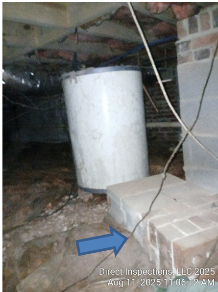
Displaced or failed
