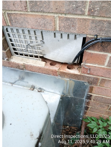
Damage by modification
