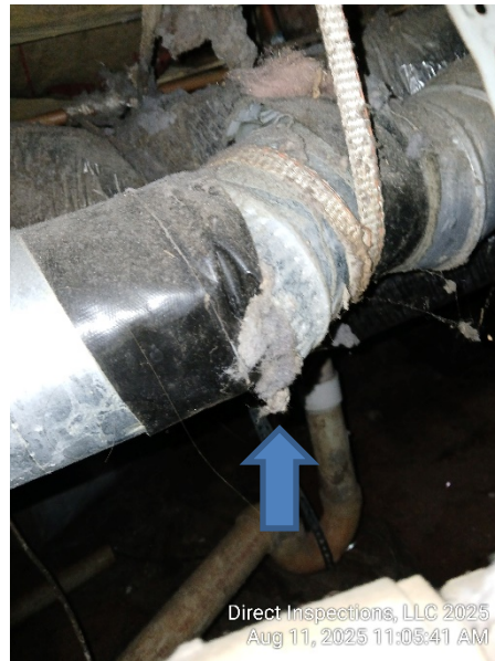
Amateur failed repairs
