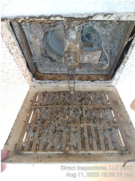
Completely clogged and broken
