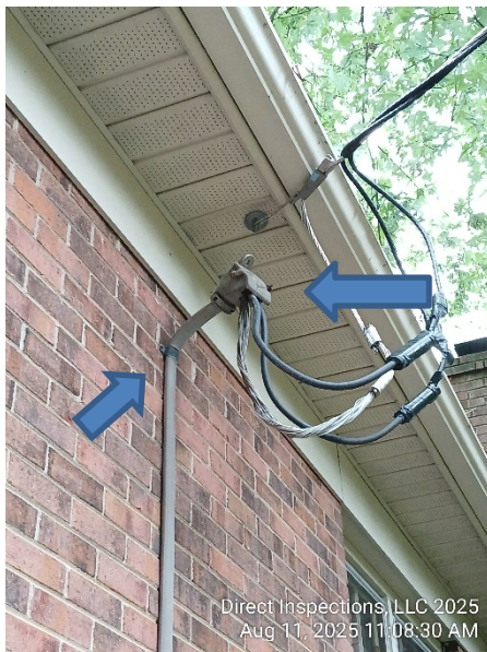
Mount failure and strap damage
