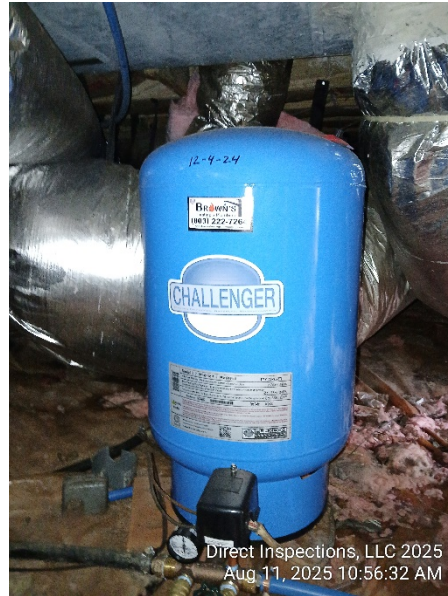
Old well system components
