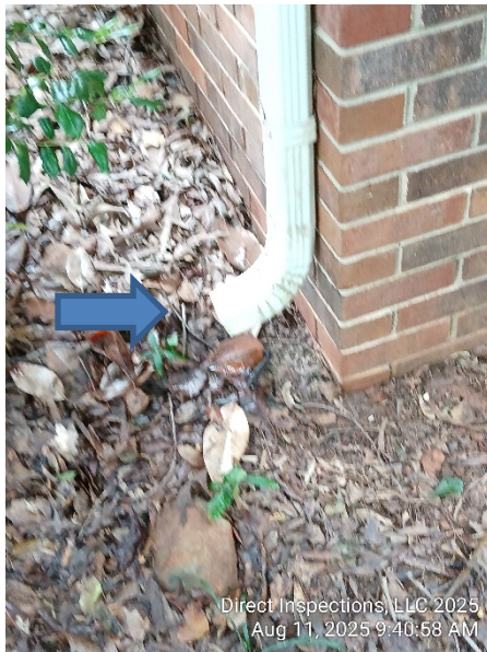
Too close to foundation
