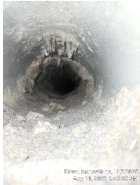
Partial clog (dryer vent)
