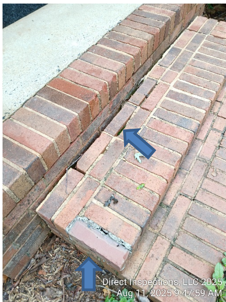
Amateur repair, missing mortar
