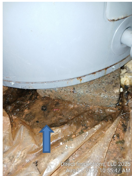
Water pooling from leak
