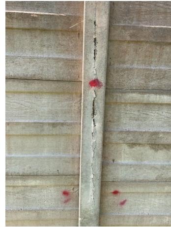
Concrete cracks and deterioration
