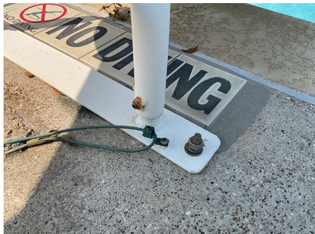
Fastener and frame rust
