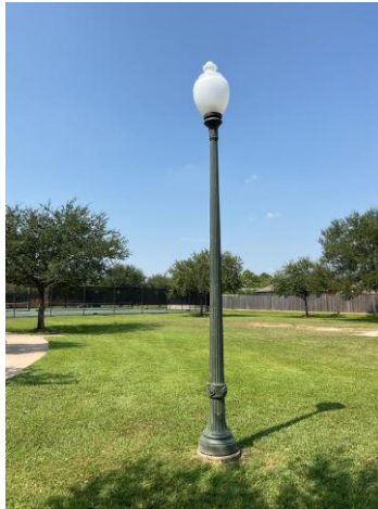
Light pole and fixture overview
