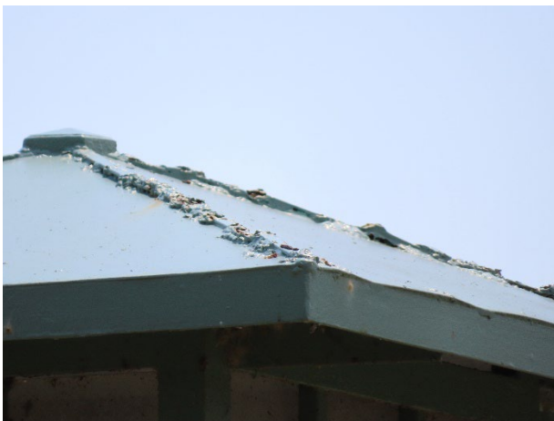
Corrosion at metal roof
