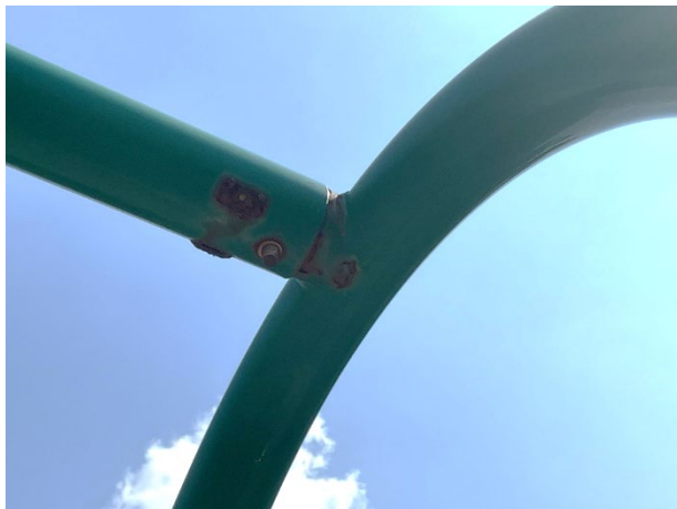
Frame rust at the pool house
