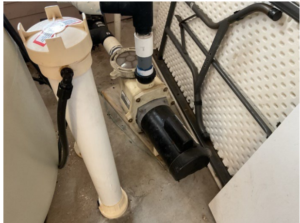
Pool mechanical equipment overview
