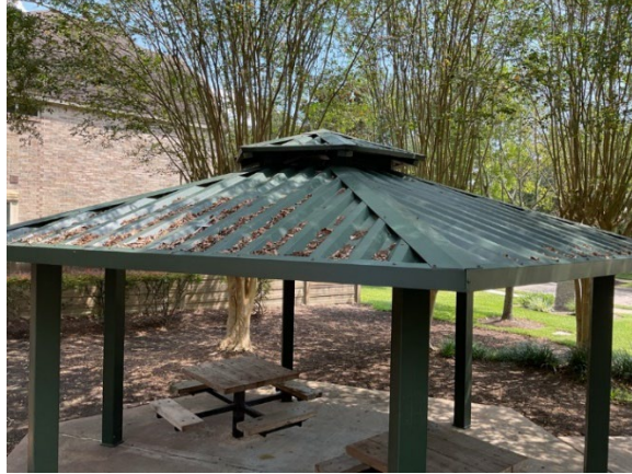
Debris accumulation at roof
