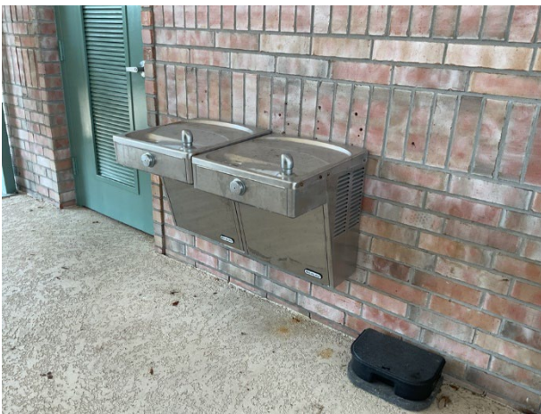
Water fountain overview
