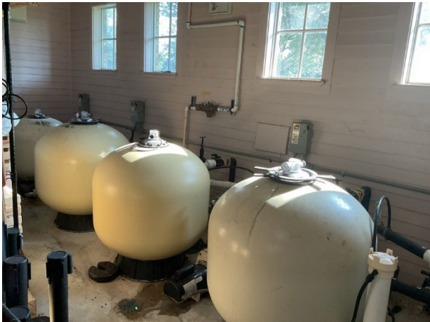
Pool mechanical equipment overview
