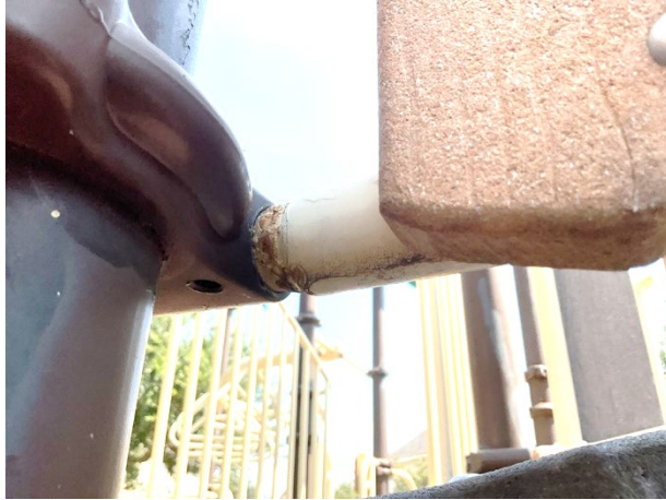
Frame rust at the pool house
