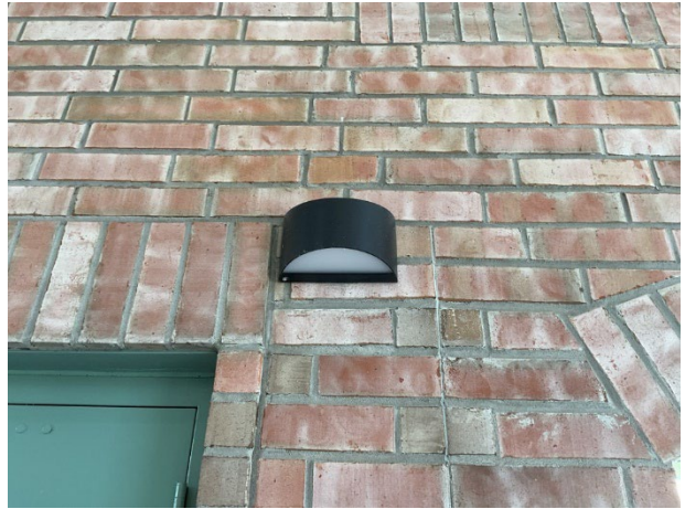
Exterior light fixture overview
