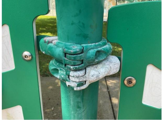
Equipment finish deterioration at the pool house
