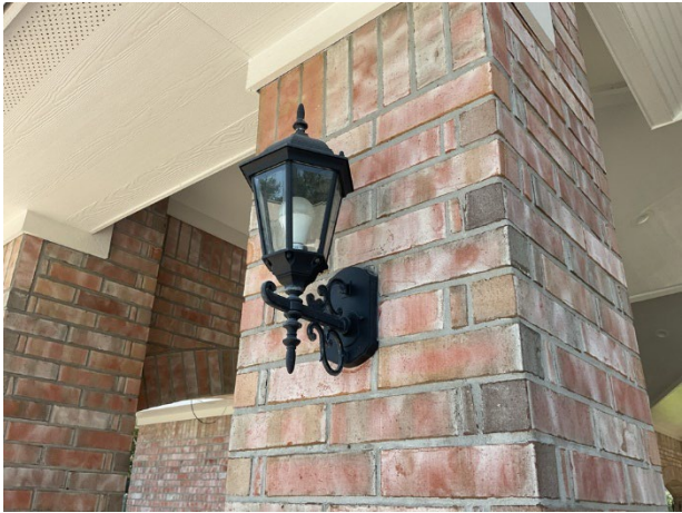
Exterior light fixture overview
