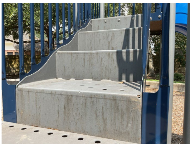
Equipment stains at Island Crossing Lane
