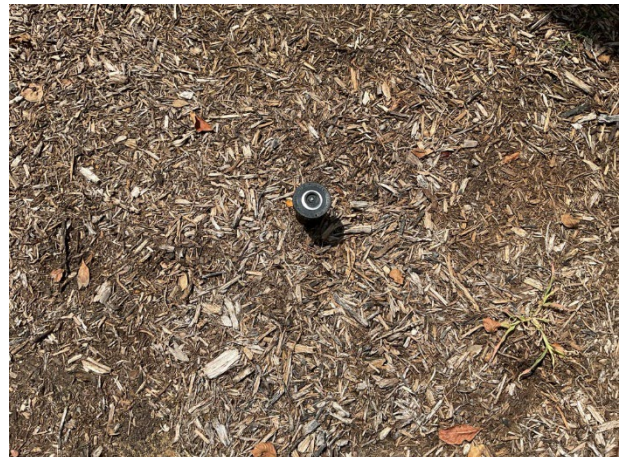
Irrigation system head overview
