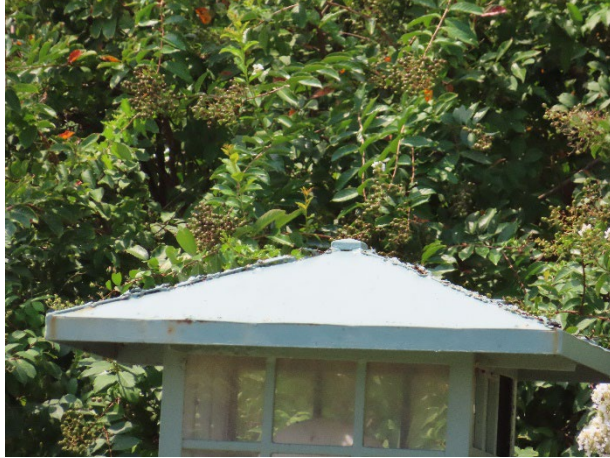
Rust at roof
