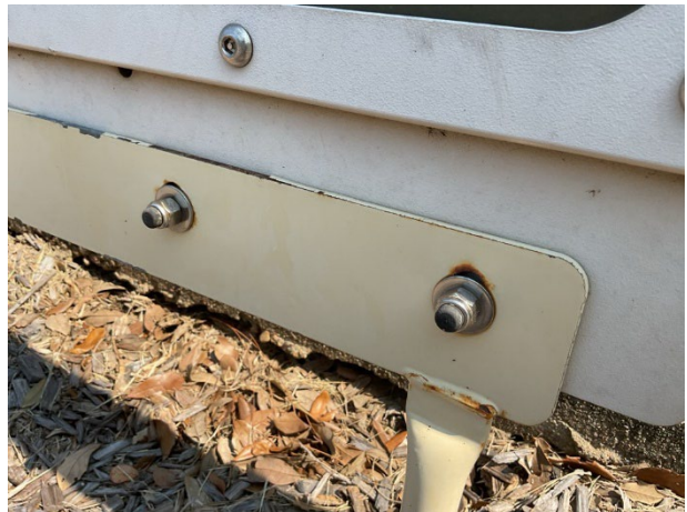
Minor frame rust and finish deterioration at the pool house
