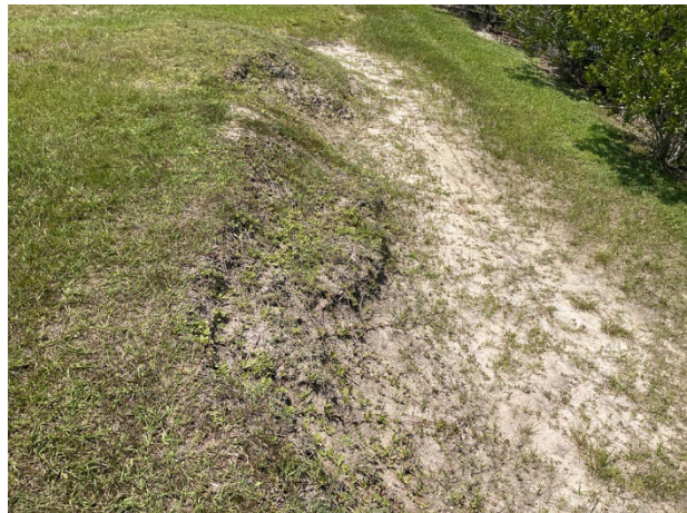
Shoreline erosion at Tucker Road Lake
