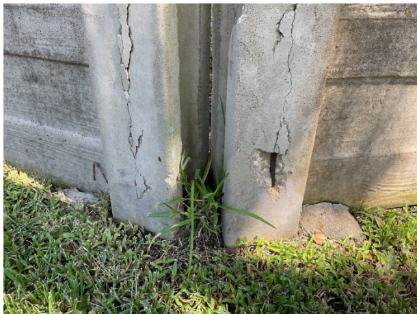
Exposed reinforcements and concrete deterioration
