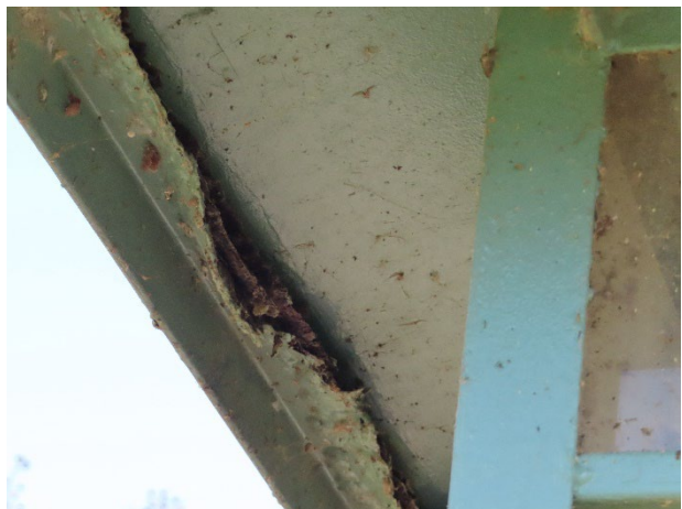
Corrosion at metal roof
