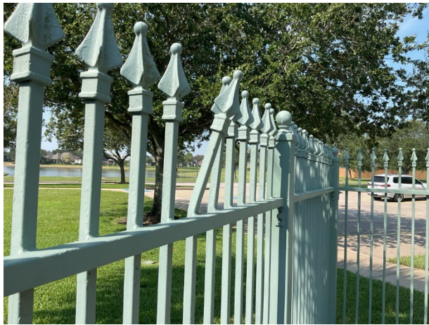
Bent fence post
