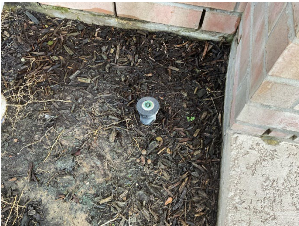
Irrigation system head overview
