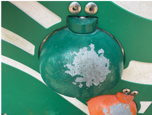
Equipment finish deterioration at the pool house
