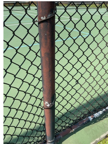
Post rust and finish deterioration
