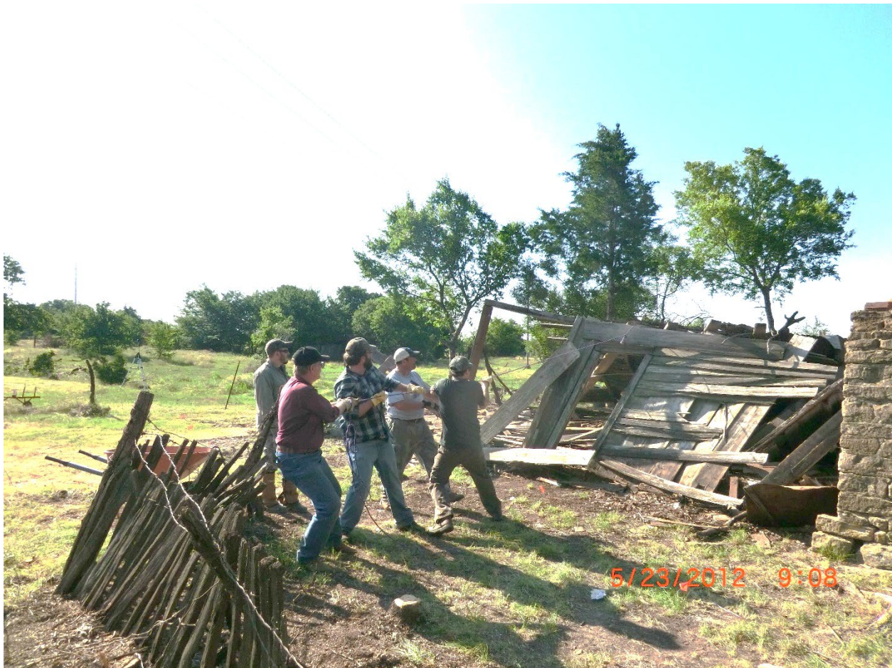
Alan leading the charge with Nick Coleman, Lee Green, Justin Boxwell, and myself on clearing the collapsed superstructure at the Redwine site (41COL228). Photo credit: CSD.
