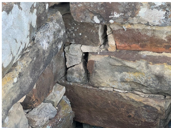
Figure 5. Photo of cistern showing grout or mortar that is cracked due to damage to structure.
