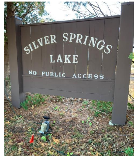
New East SSL LED Entry Light:
