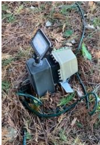
East SSL - New LED floodlight
