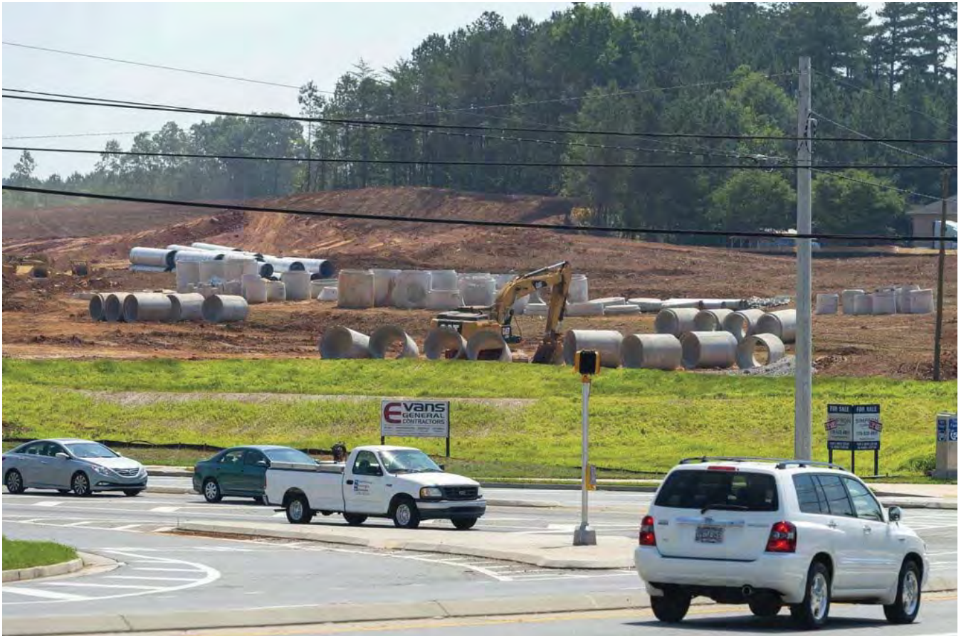
Grading work takes place at a 44-acre lot at the intersection of Lanier Islands Parkway and Atlanta Highway in Buford on Friday, June 8, 2018, which will be the site of an industrial park. 985 Lanier Logistics will be across from a QuikTrip convenience store. - photo by David Barnes
