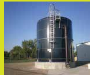
Water supply to overhead tanks
