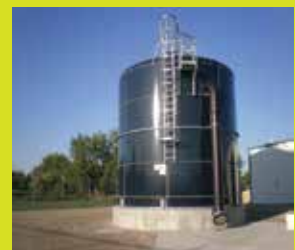
Water supply to overhead tanks
