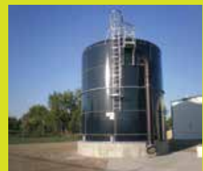
Water supply to overhead tanks
