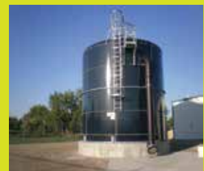
Water supply to overhead tanks
