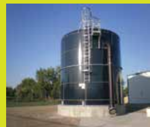
Water supply to overhead tanks
