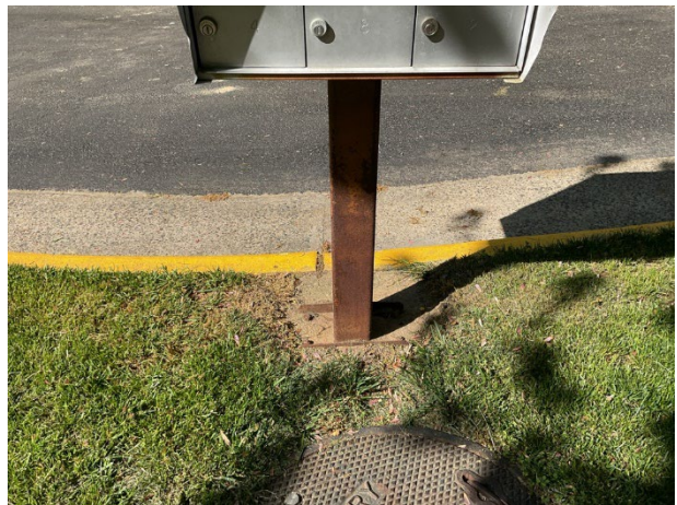
Original mailbox station – Note: rust
