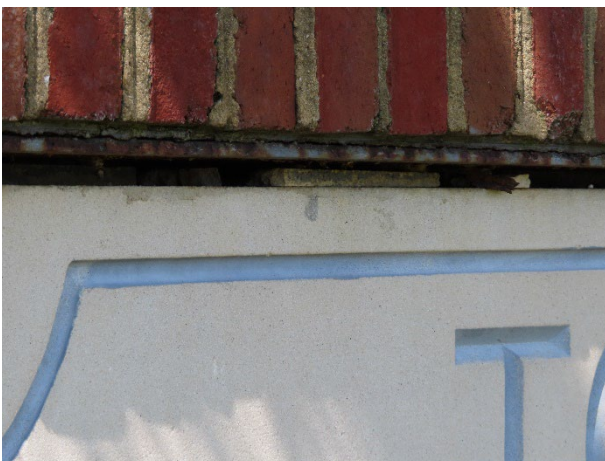
Mortar deterioration and lintel rust
