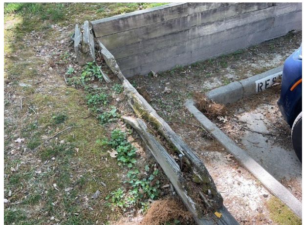
Wood rot at Peter Roy Court
