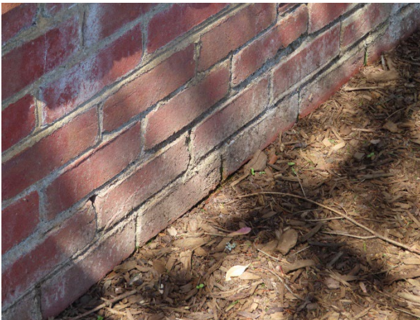
Mortar deterioration and efflorescence
