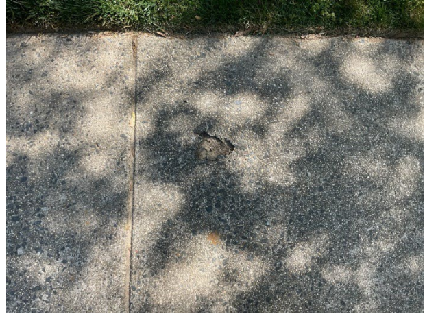
Concrete sidewalk damage
