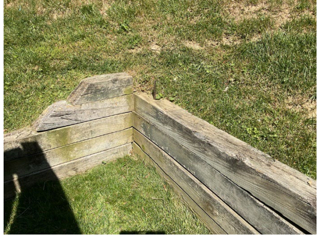
Missing timber tier behind 9410 William Kirk Lane
