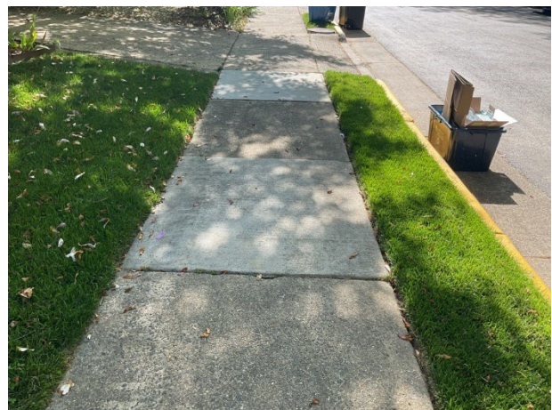
Concrete sidewalk previous repairs
