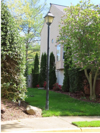
Light pole and fixture overview
