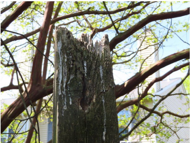
Wood post deterioration
