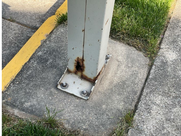
2006 mailbox station – Note: Minor rust
