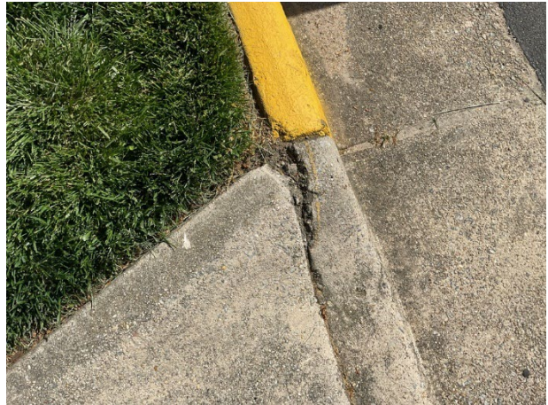
Concrete curb damage
