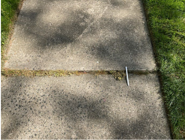
Sidewalk trip hazard near unit 9458
