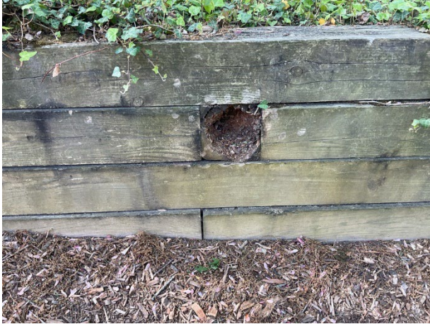
Wood rot at Peter Roy Court
