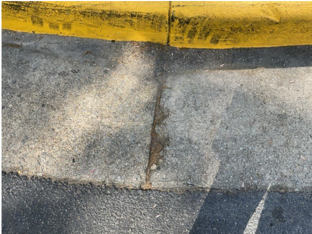
Concrete gutter damage
