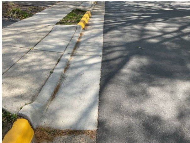
Concrete curb and gutter previous repair
