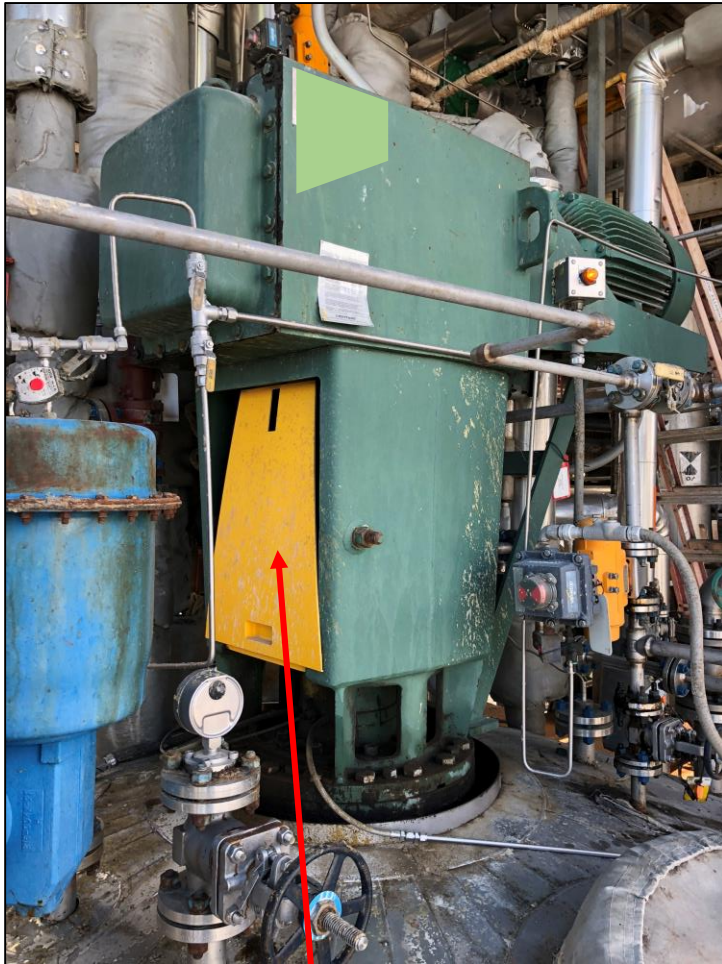
BEFORE DOOR MODIFICATIONS (Plastic Door)
