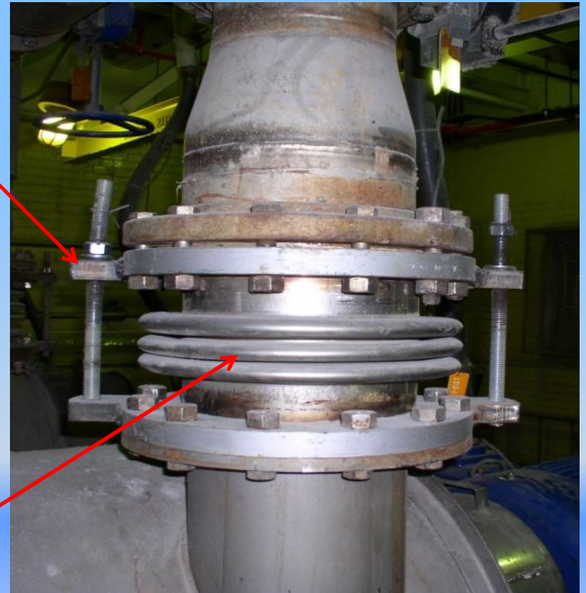
Figure 12. Blower LS 10 Blower Discharge Connection, Bellows Collapsed.
