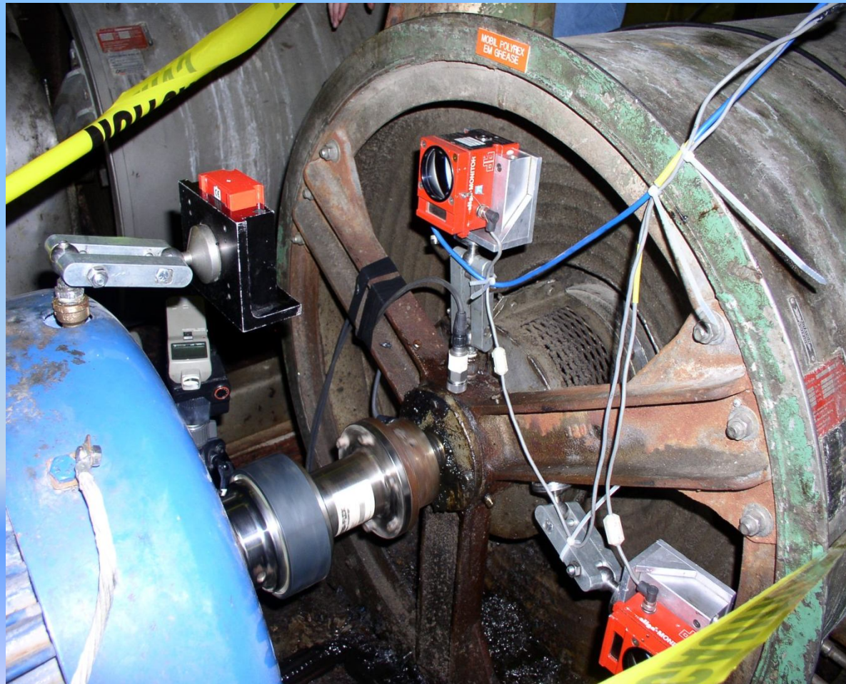
Figure 14. DB 19 With Laser Alignment and Vibration Sensors Attached.
