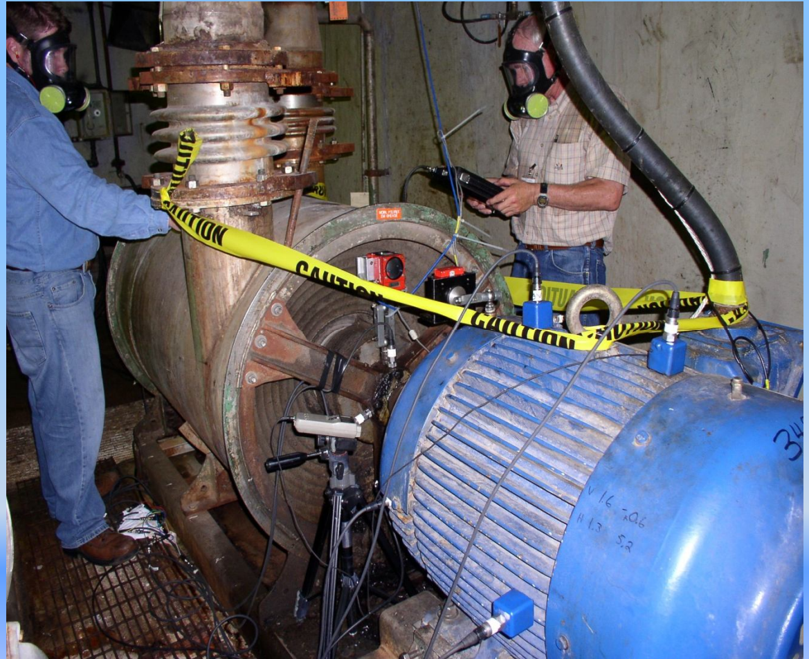
Figure 33. Laser Alignment Equipment, Ludeca Permalign, Ref 7 Installed on the Motor and Blower.
