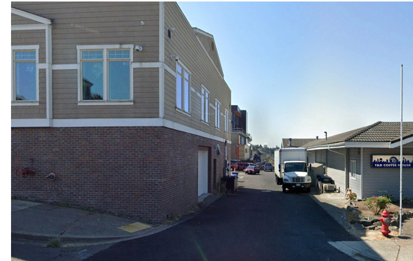
Utility undergrounding completed in Des Moines Theater alley at S 223rd St
