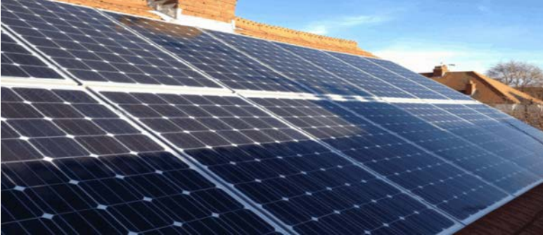
Fig. 2. Occurrence of shading in a rooftop solar PV system
