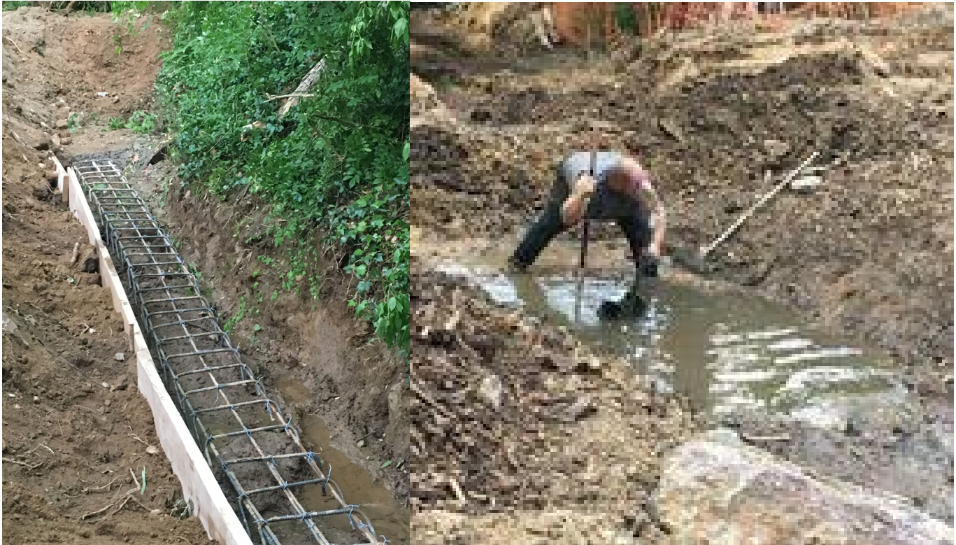
Rebar is used to protect buried sewer pipes from heavy equipment used during the restoration process as workers build the riffles and pools to help limit future storm water damage to the creek and surrounding banks.
