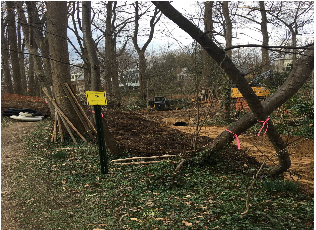
Storm water run-off has weakened tree roots in the Park. Some trees have had to be removed as part of the restoration work.
