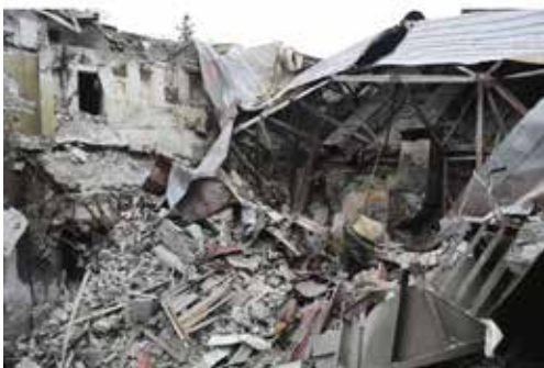
FILE - Rubble from the damaged Donetsk Academic Regional Drama Theatre sits after the March 16, 2022, bombing in Mariupol, Ukraine, in an area now controlled by Russian-backed separatist forces, on Monday, April 4, 2022. The bombing of the theater, which was used as a shelter, stands out as the single deadliest known attack against civilians to date in the Ukraine war. (AP Photo/Alexei Alexandrov, File)
