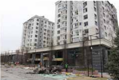
Damaged building of the Continent housing complex pictured in the city of Bucha on April 5, 2022 (The Kyiv Independent)
