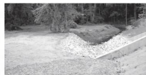
A culvert under North Charles Street north of Cold Spring Lane near Johns Hopkins University has been completed and the sidewalk secured.
