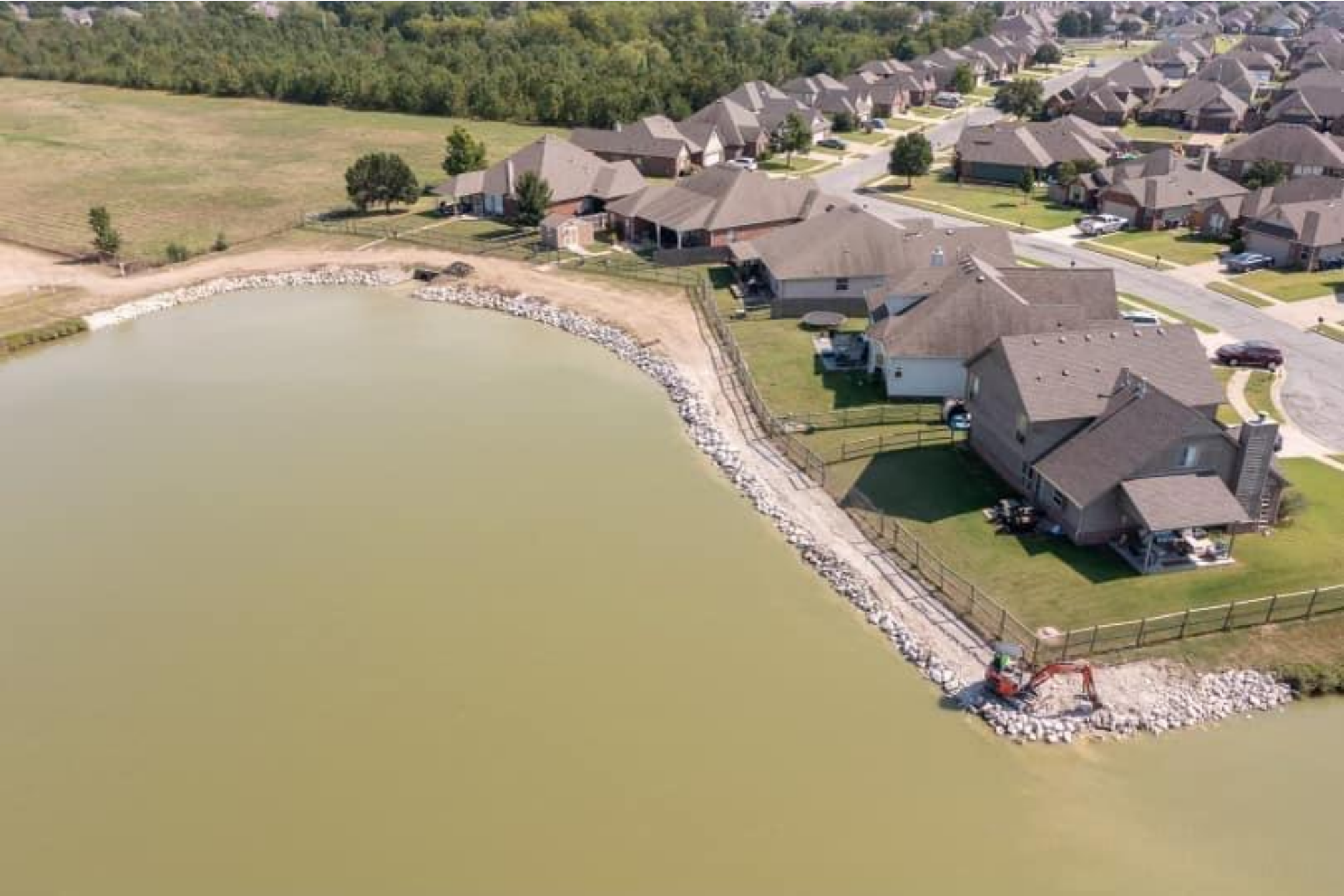
Southeast Pond Bank Repair completed by Eagle Eye Construction, Inc and before sod was laid
