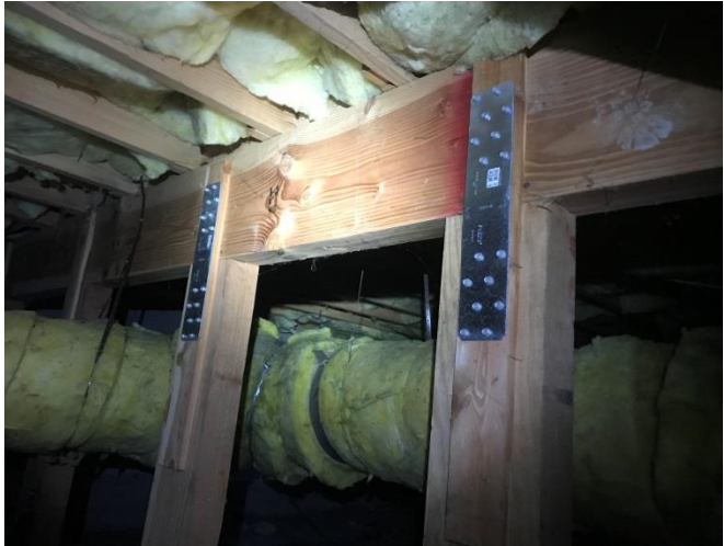
Main support beam attached to vertical supports that go to 12 concrete piers. This important structural beam that the rest of the house is built upon, was barely attached with a thin piece of 1 inch wood to the vertical posts shown here, and the posts were NOT attached to the concrete piers. These act as vertical load bearing support only and in the event of an earthquake, the houses' mass will shift from side to side freely. If these wooden supports crumble, the house is going to sag downward in its middle badly. We added these metal plates to join the beam to the vertical supports.
