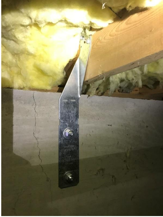
Example of a floor support beam being attached to the foundation. We did this in numerous locations.
