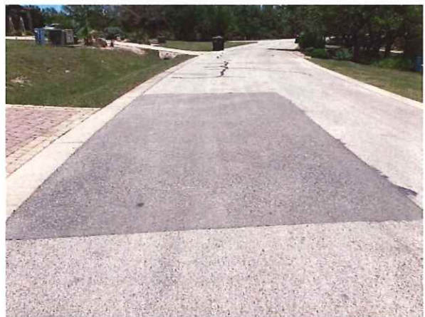
Previously patched section
