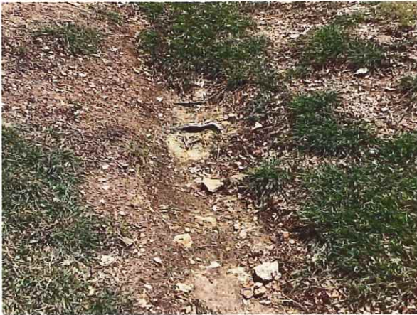
Erosion at swale
