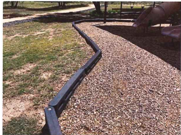
Safety surface and border
