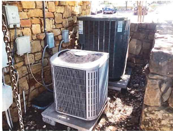
Split system condensing units
