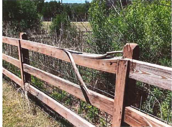
Fence picket damage
