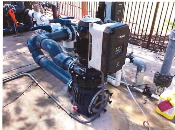
Pool pumps and controls
