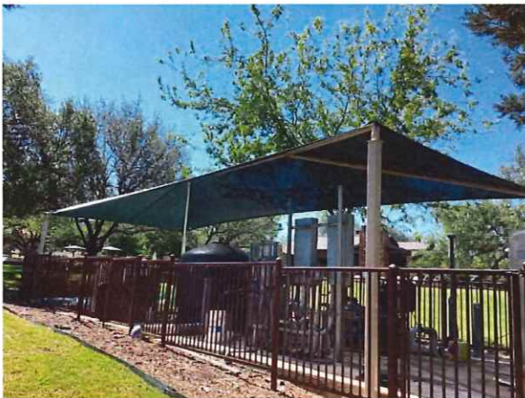
Shade structure above pool mechanical equipment
