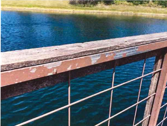
Finish deterioration at railing
