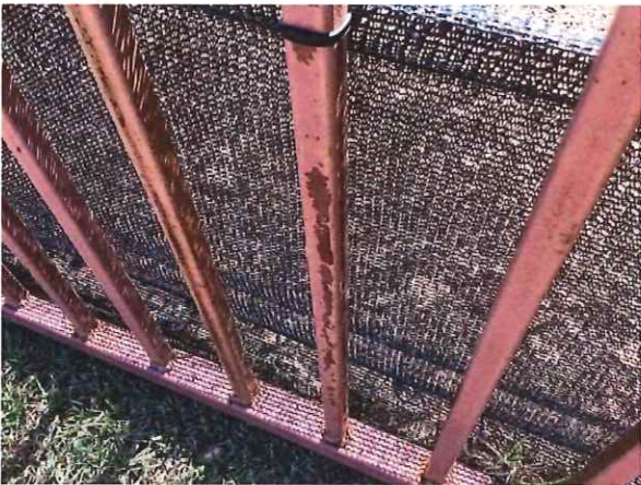
Fence finish deterioration
