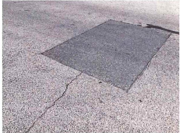
Pavement cracks and previously patched section
