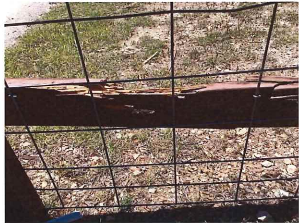
Fence picket damage
