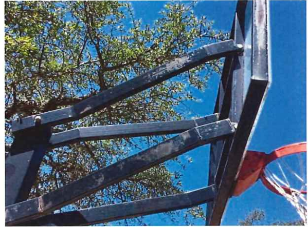
Rust at basketball goal
