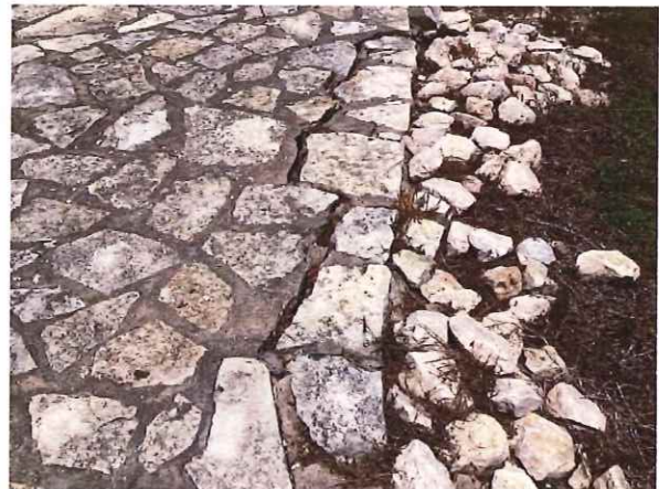
Flagstone trail deterioration
