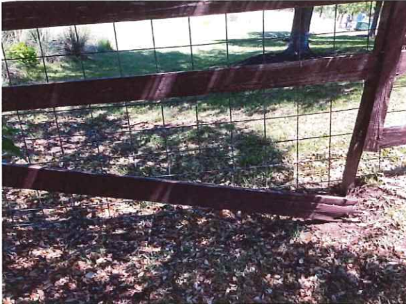
Fence picket damage
