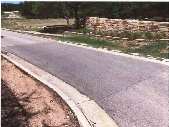
Previously patched section
