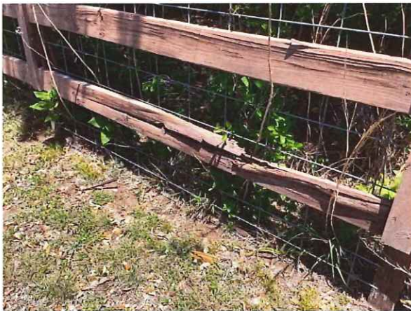
Fence picket damage
