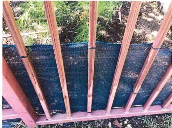
Fence finish deterioration
