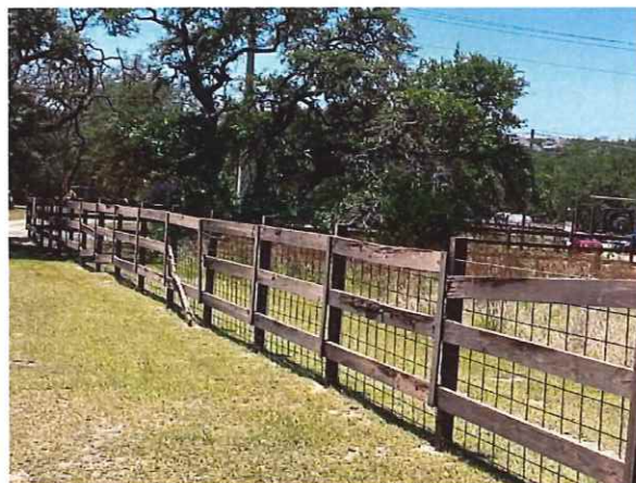
Fence picket damage
