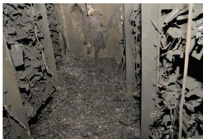
Fire damage to starboard battery room
