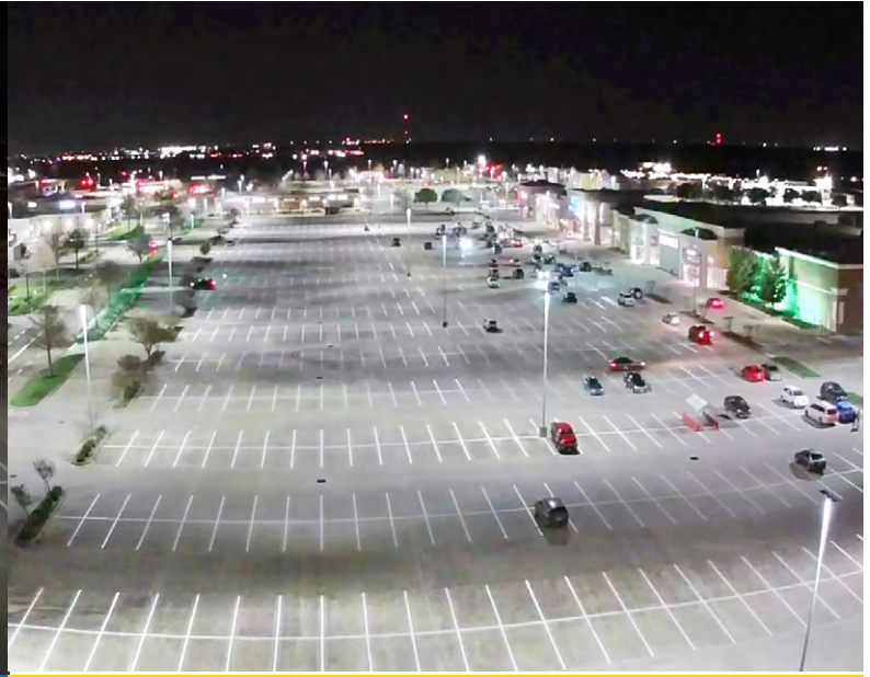
AFTER: NEW LED PARKING LOT LIGHTING
