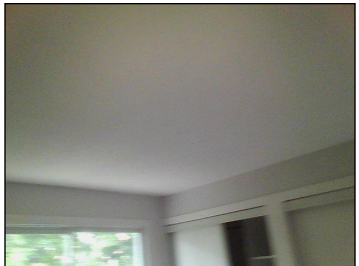
52. Inspection was performed by thermal imaging.
