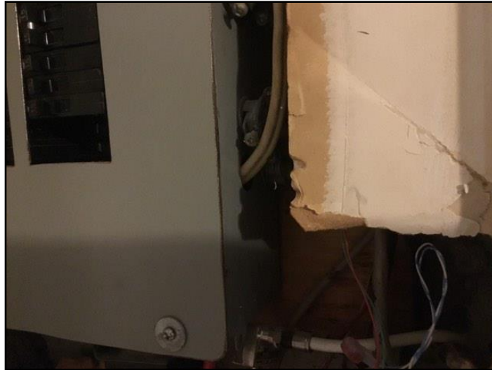
21. Not well secured
