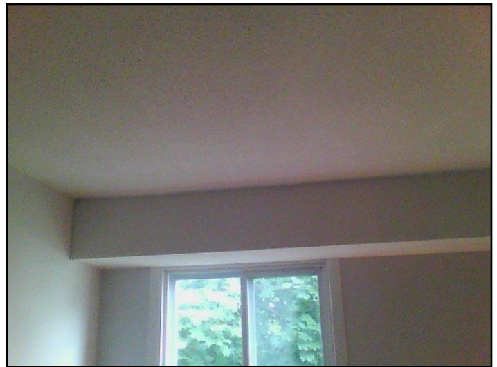
46. Inspection was performed by thermal imaging.
