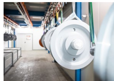
New drying facility with waste heat recovery
