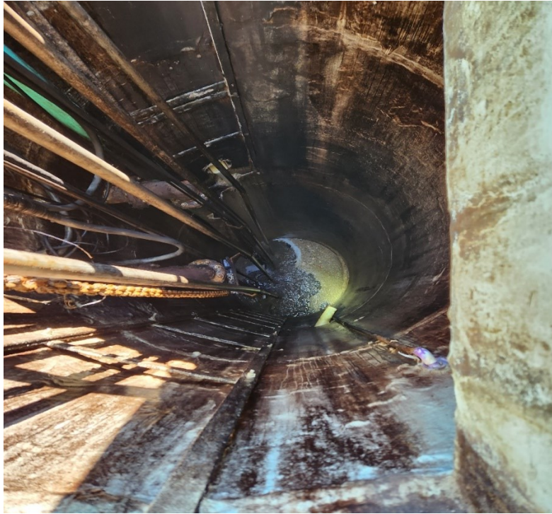
Above – wet-well at 16 Barre Drive Pumping Station
