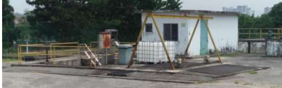
Fig. 1: Dosing tanks at the inlet of the STP
