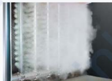
Dry steam humidification
