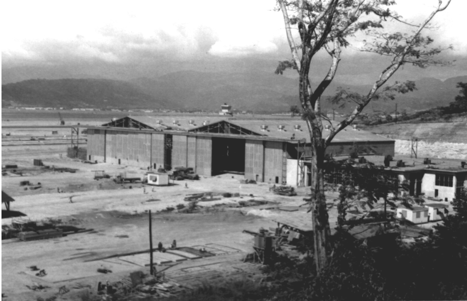
Left: Hangars and office building under construction at Naval Air Station, Cubi Point, Subic Bay, early 1956.
