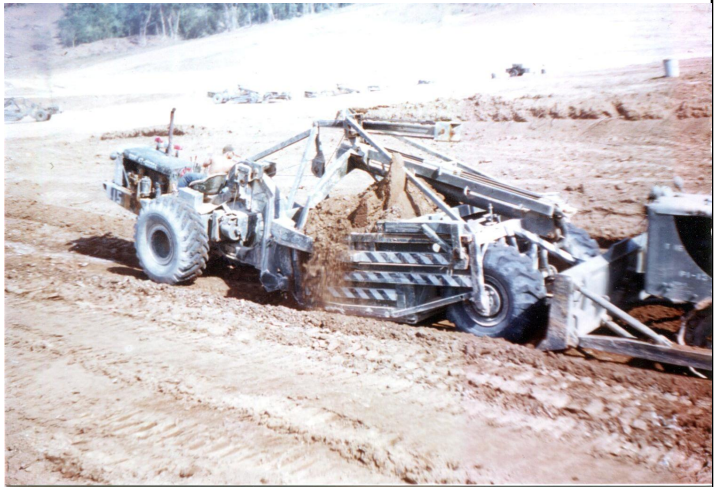
Above, all three pictures: Cat and pan operation building the airstrip at Cubi Point, Subic Bay, P.I. April 1952
