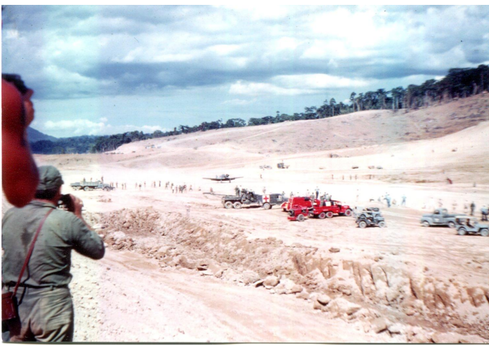
Above: First airplane to land on the Cubi Point airstrip, under construction. May 1952
