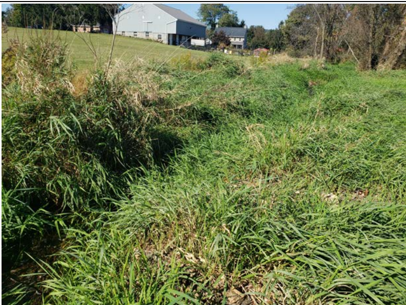
Photo 3. Upstream section eroded left bank
