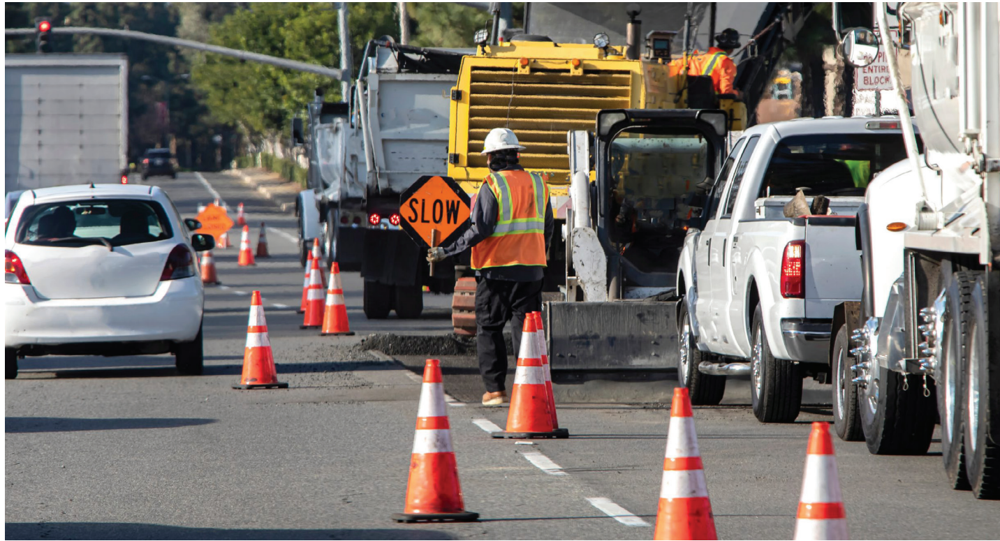
A worker holds a sign advising motorists to go slow through the temporary construction area.
