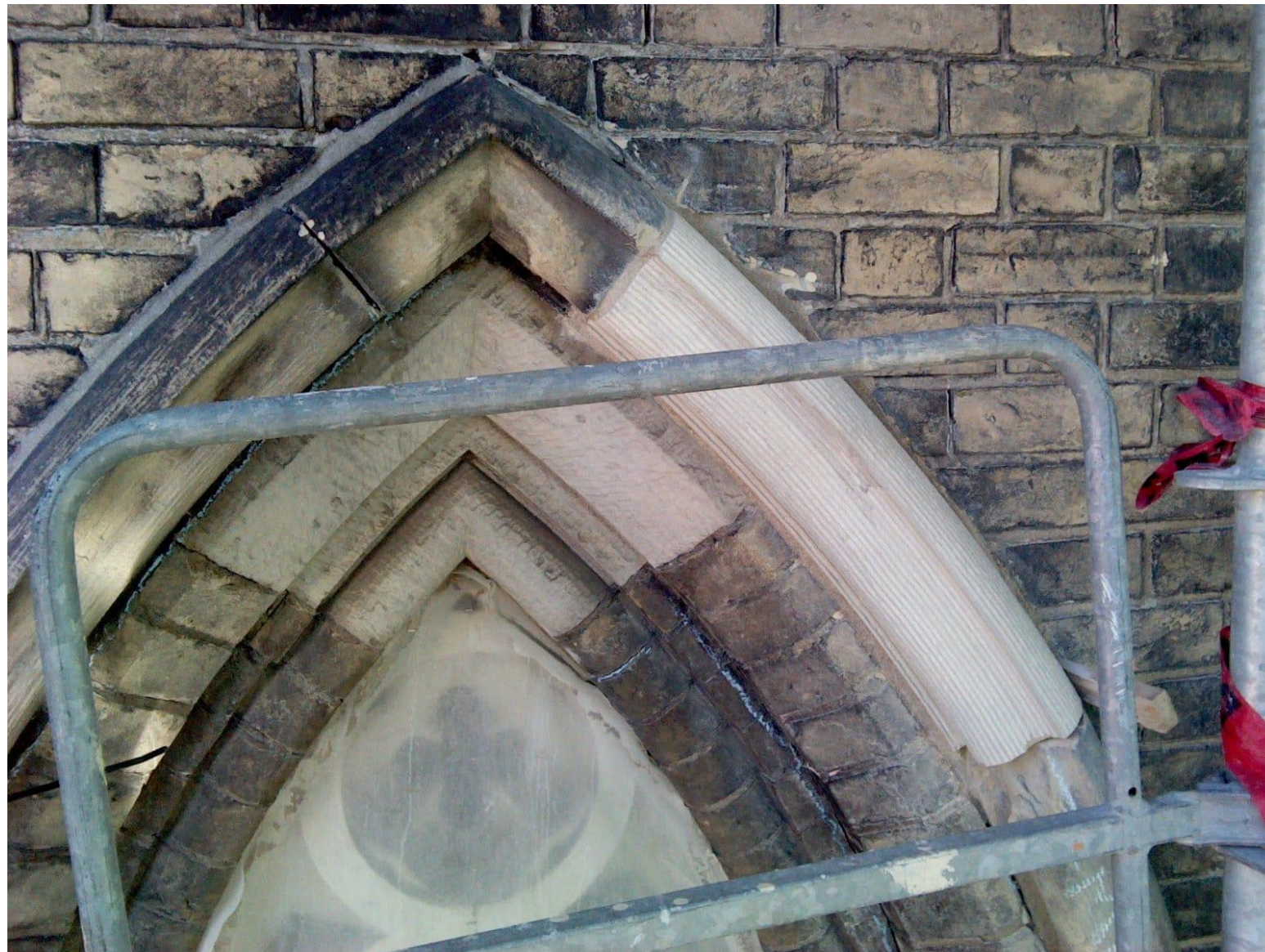
Picture above and to right: New Stone hood molding sections on Gothic arch.
