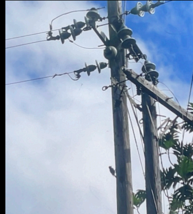
ALTERED STRUCTURAL INTEGRITY
