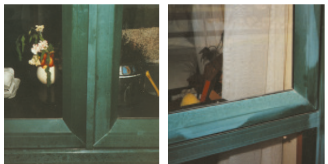
Examples of solvent misuse on aluminium joinery, showing deterioration of powder coating after 3 years.
