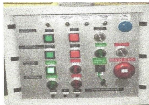
Fig. 11 The Control Panel
