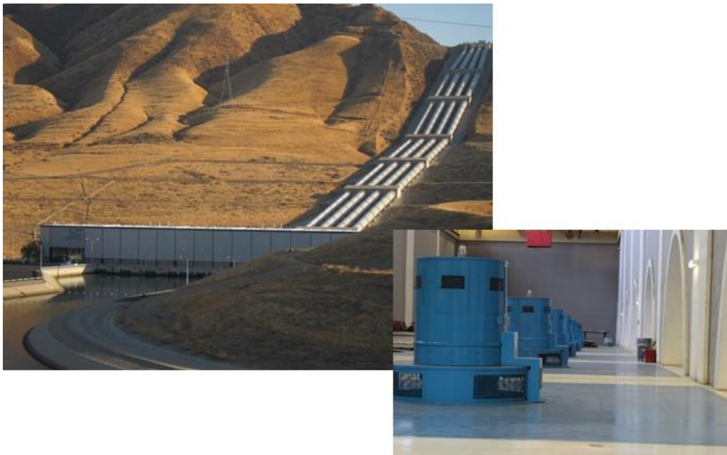
Figure 2: Chrisman Pumping Plant (Left) and Edmonston Pumping Plant (Right)
