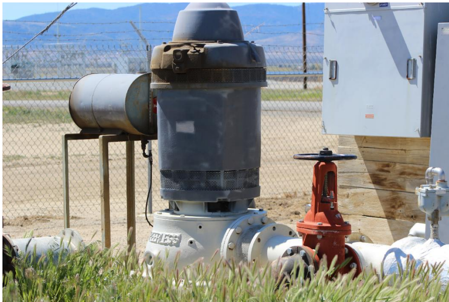
Figure 14: A Groundwater Well at Willow Springs Water Bank
