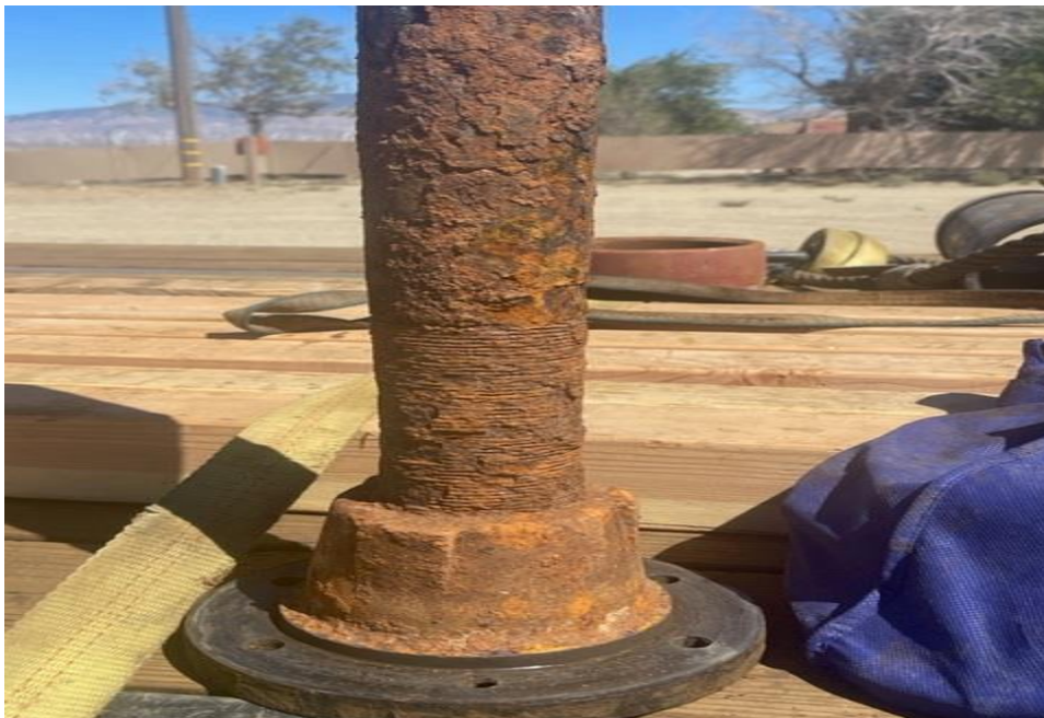
Figure 11. Severe Rusting on Well Pipes
