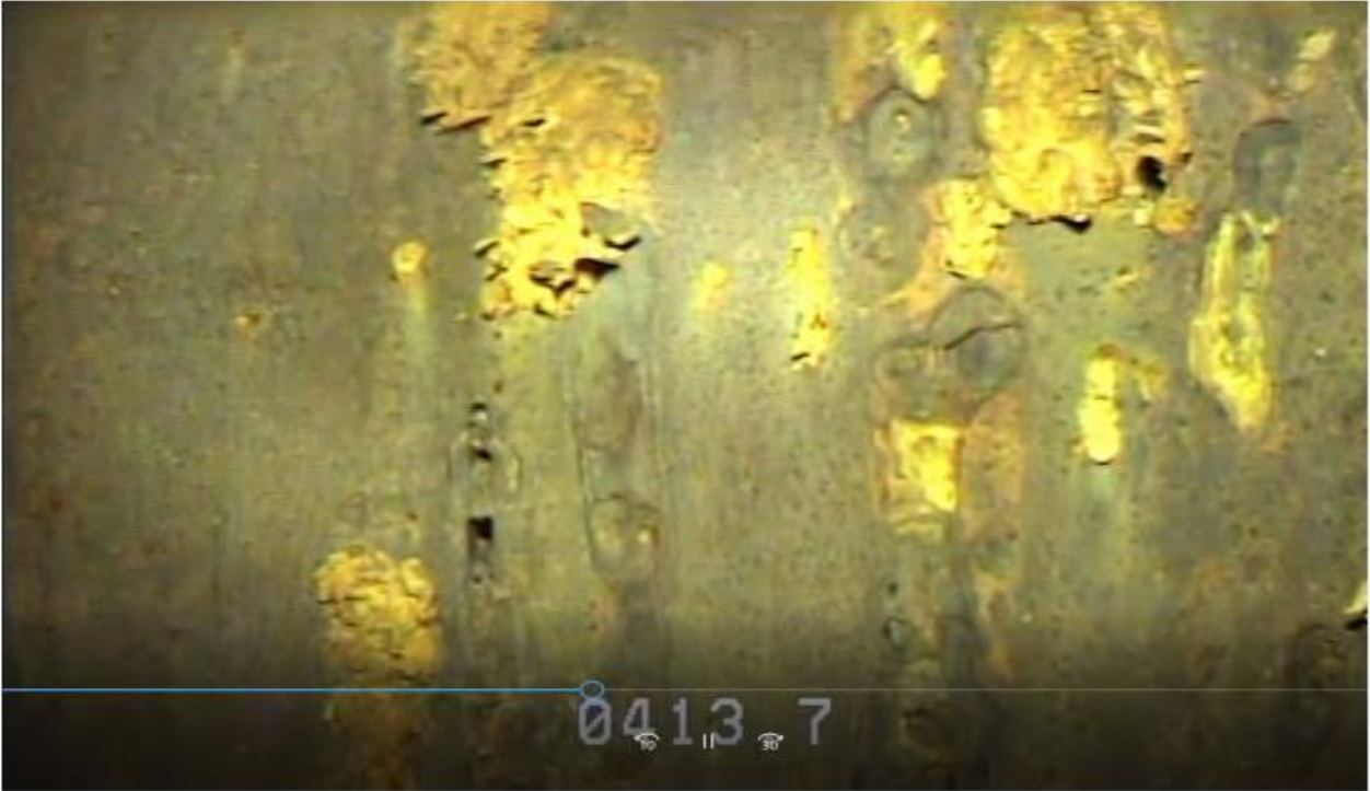
Figure 5. Biofouling with some open casing perforations at 414 ft deep
