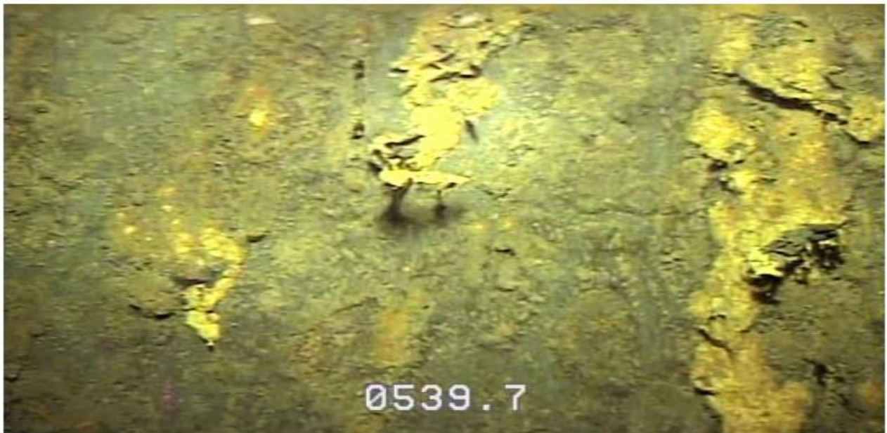
Figure 6. Completely blocked casing perforations at 540 ft deep.
