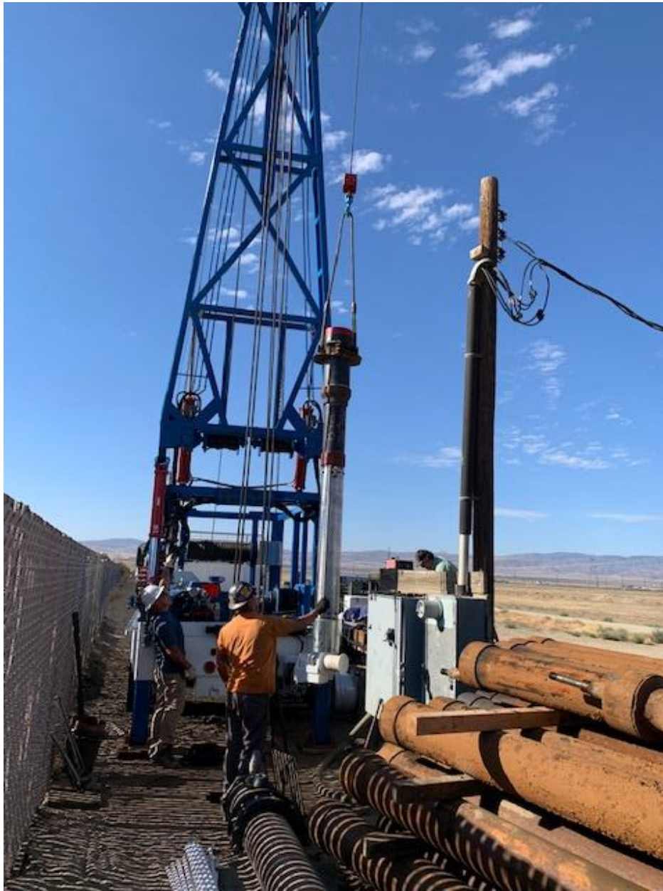
Figure 14. APH Valve Installed at Bottom of Pipe Column
