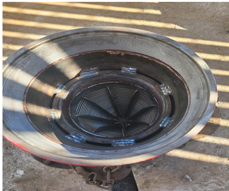
Figure 13. Screen above APH Valve
