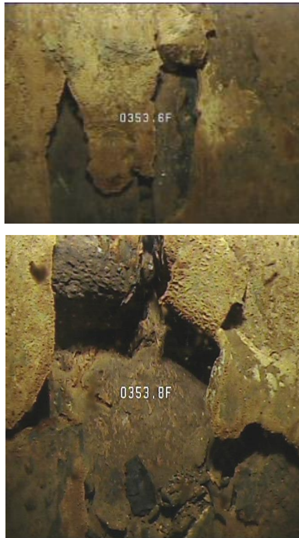
Figure 9. Patch and Obtrusions at 353 Ft.
