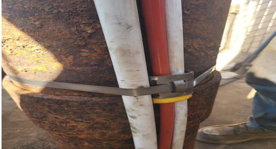
Figure 10. APH Valve Hydraulic Hoses on Exterior of Well Pipe
