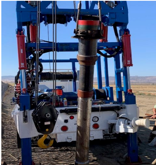
APH Valve Installed Below Pump Bowls
