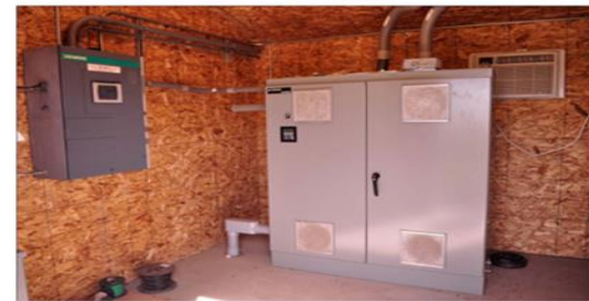
200 HP MOTOR STARTING VFD & 100 HP REGENERATION VFD WITH LOCAL CONTROL PANEL.
