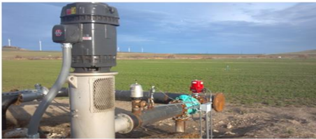
200 HP MOTOR WITH VERTICAL LINE SHAFT PUMP - 8" PIPE, AQUIFER LEVEL 520 FEET BELOW LAND SURFACE.
