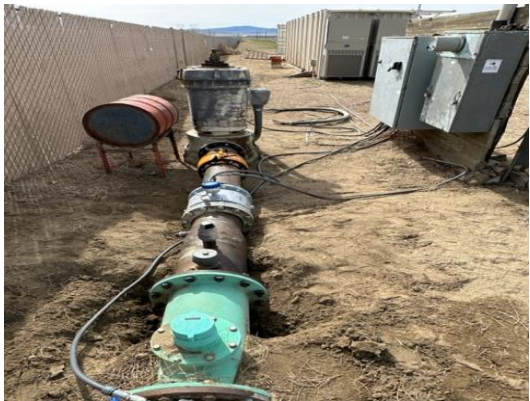
Existing Well Pump to APH
