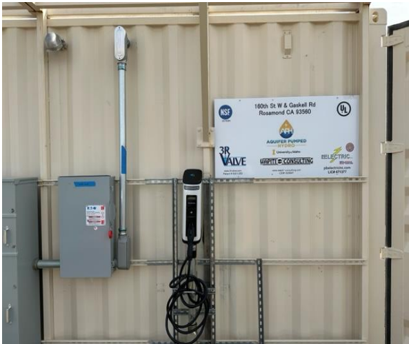
APH Container with EV charger
