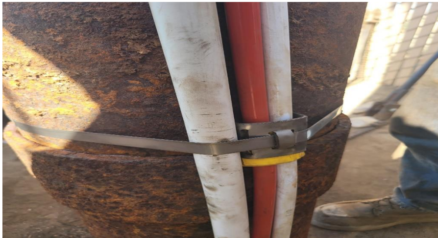
Figure 7. APH Valve Hydraulic Hoses on Exterior of Well Pipe
