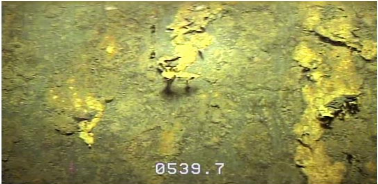
Figure 3. Completely blocked casing perforations at 540 ft deep.
