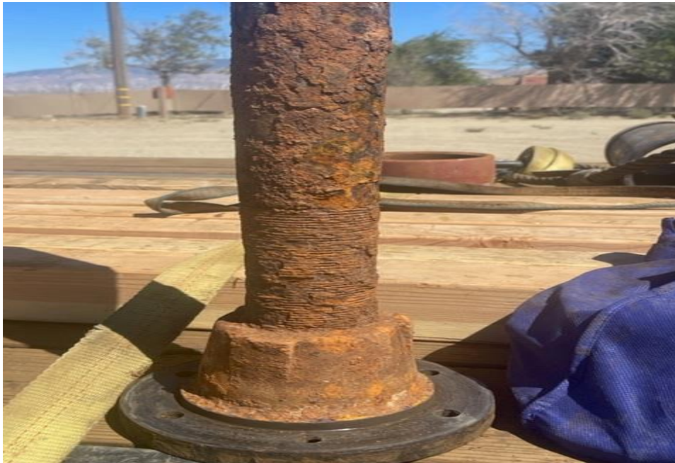
Figure 8. Severe Rusting on Well Pipes
