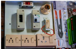
One of the 500 electrical switchboards fabricated to restore power to those affected by Kerala floods
