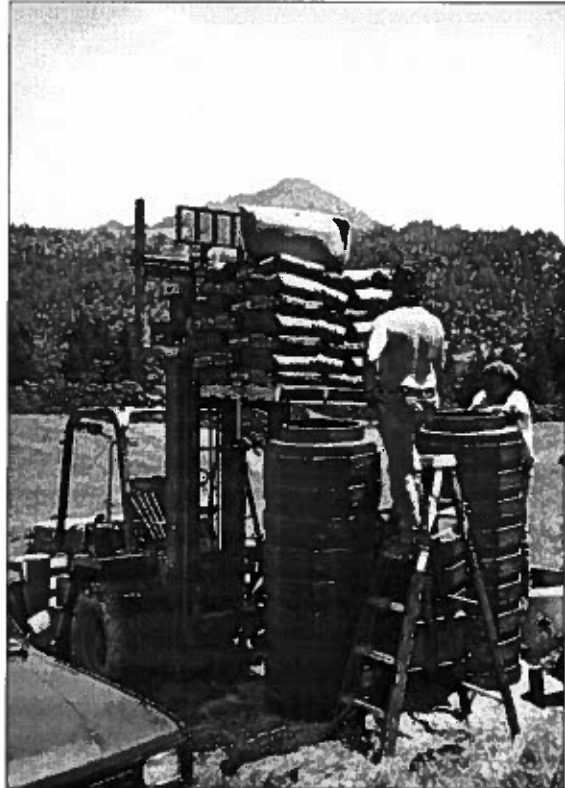
Loading bagged sand into the two tanks of a slow sand filter.
