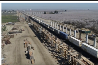
The Wasco Viaduct , under construction in 2020. A BNSF freight train is passing underneath the then-future pergola.
