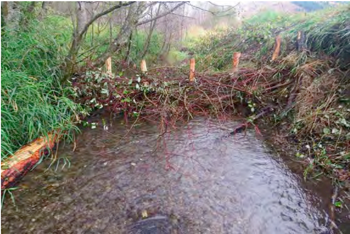
Figure 75: Pilings woven with live red oyster dogwood, some of which was planted directly into the exposed bank to facilitate resprouting
