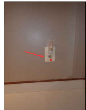
Missing GFCI Outlet
