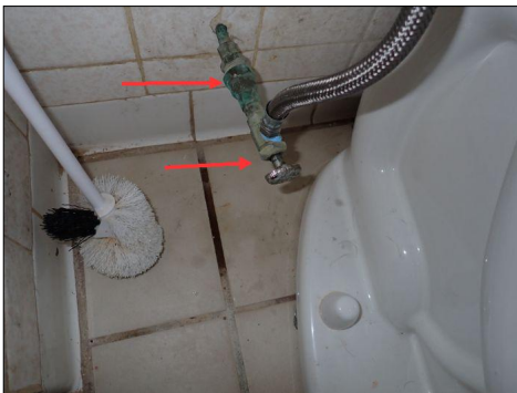
Toilet Supply Valve
