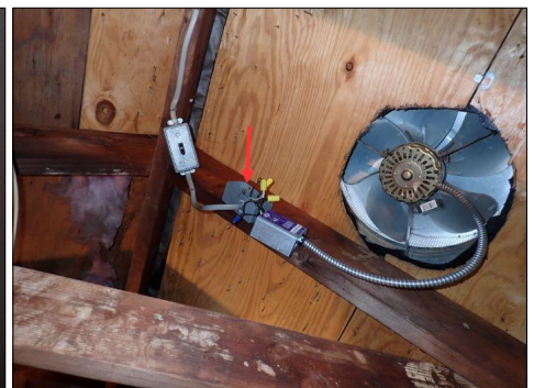
Open Electrical - Attic
