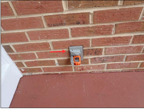
Missing GFCI Outlet
