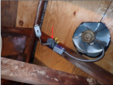
Open Electrical - Attic
