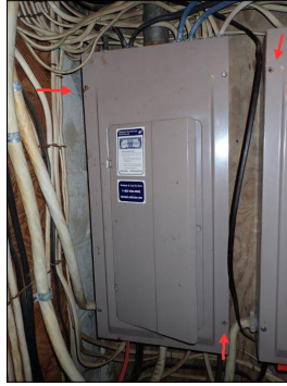
Main Electrical Panel
