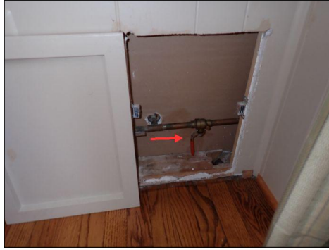
Front Hose Bib Shutoff
