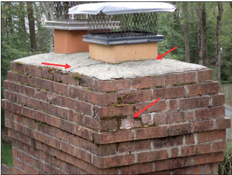
Chimney - Cracked Brick / Mortar
