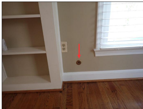
Missing Dante Valve Key
