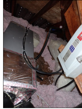
Heat Pump - Unit #2
