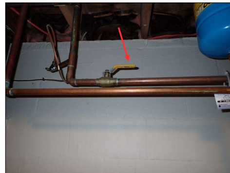
Water Heater Supply Valve
