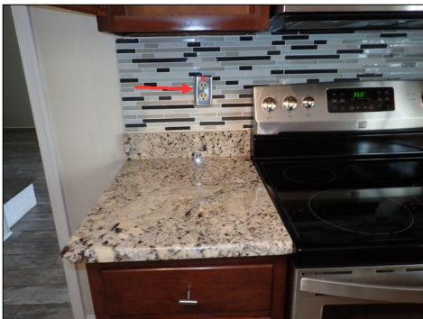
Missing GFCI Outlet
