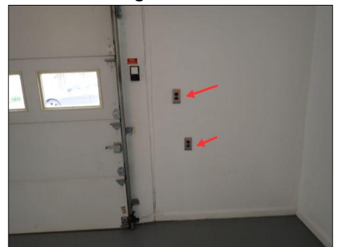
Missing GFCI Outlets
