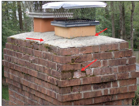
Chimney - Cracked Brick / Mortar
