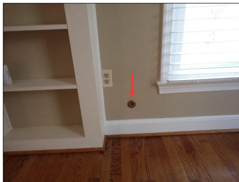
Missing Dante Valve Key
