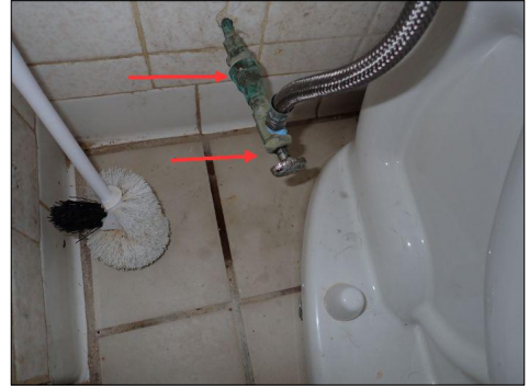
Toilet Supply Valve
