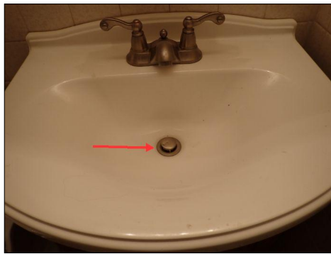
Bathroom Sink Drain
