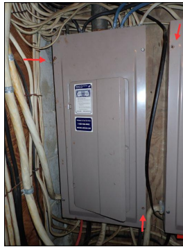
Main Electrical Panel
