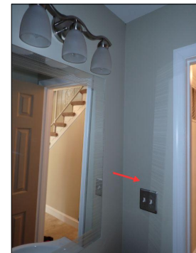
Missing GFCI Outlet
