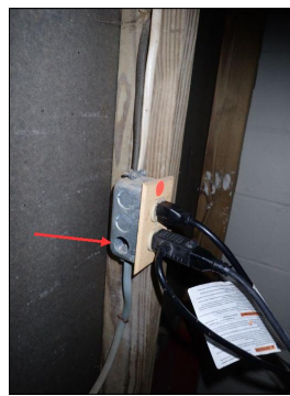
Open Electrical - Basement
