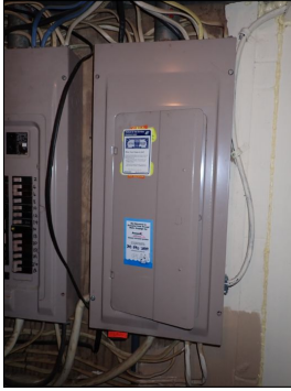
Main Electrical Panel
