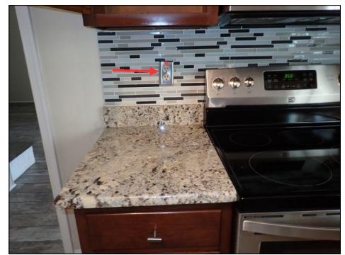
Missing GFCI Outlet
