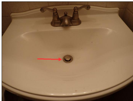
Bathroom Sink Drain
