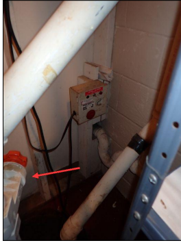
Ejection Pump On/Off Valve
