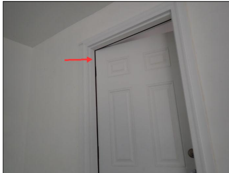
Garage to Home Door
