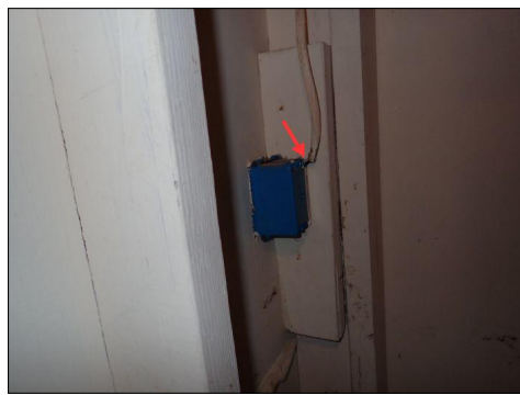
Open Electrical - Basement
