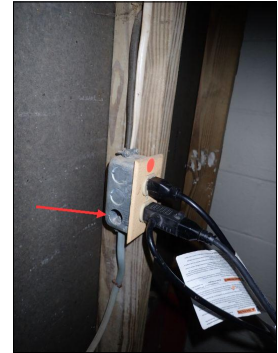
Open Electrical - Basement
