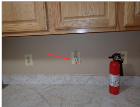
Missing GFCI Outlet
