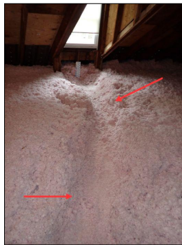
Missing Attic Insulation
