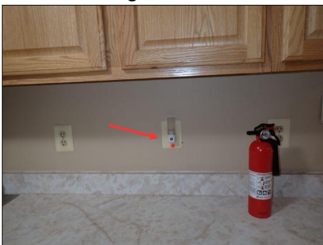
Missing GFCI Outlet
