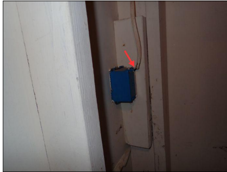
Open Electrical - Basement
