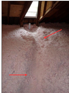
Missing Attic Insulation
