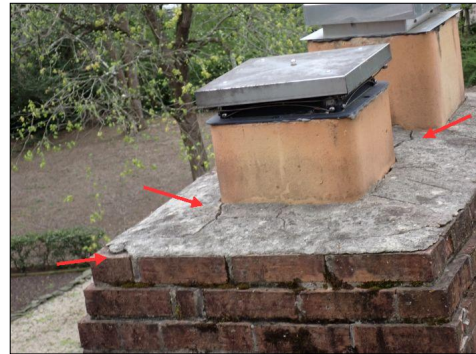
Chimney - Cracked Brick / Mortar
