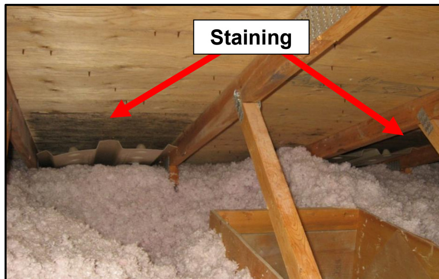
Figure 1: Staining (mold) at soffit vents in a recently constructed wood-framed attic
