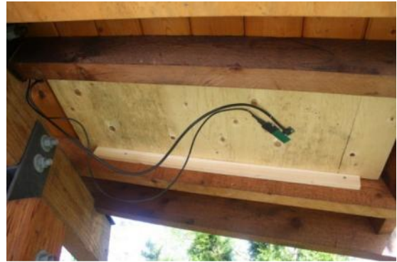
Photo 4: Mold growth on the plywood sample that is decoupled from the asphalt singles by a thick wood deck and 25 mm extruded polystyrene insulation.
