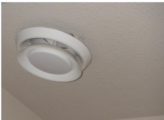
Photo 10: Fresh Air Grill with Air Leakage Path
