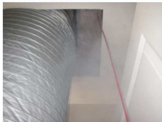
Photo 11: Air Leakage at Attic Hatch during Testing
