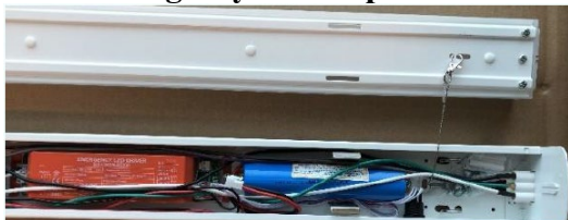
Emergency Back-up Driver
