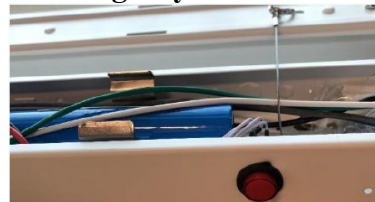
Emergency Test Button
