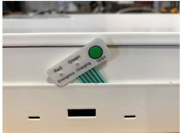
Emergency Test Button
